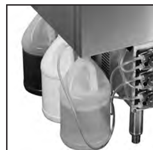
Detergent, Sanitizer, and Rinse Aid Containers
